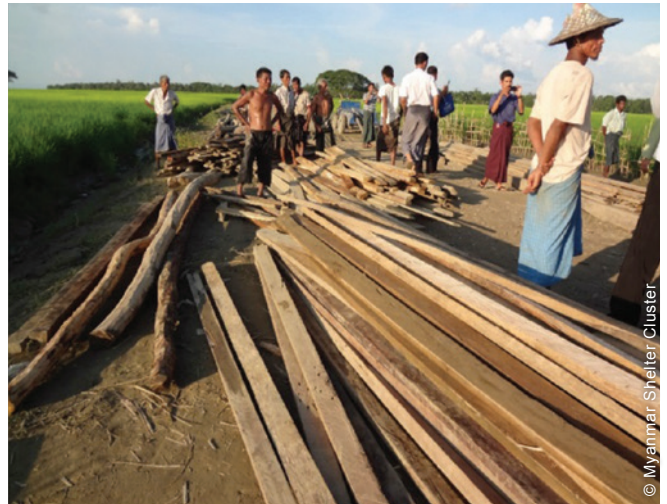
© Myanmar Shelter Cluster Construction materials were supplied by the government to rebuild the houses of IDPs affected by the violence (Thi Kyar IDP Camp, Mrauk-U Township).
