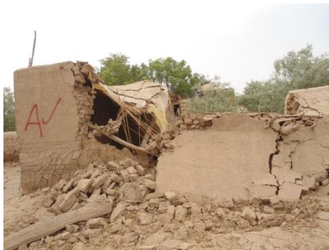
Category A (Fully Destroyed) Khwaja du Koh, Jawzjan. (Photo: People in Need)
