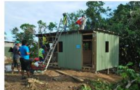
Building Back Safer 'Training the Trainers' pilot program held in May by Shelter Cluster Fiji and Habitat for Humanity Fiji (Source: Shelter Cluster)
