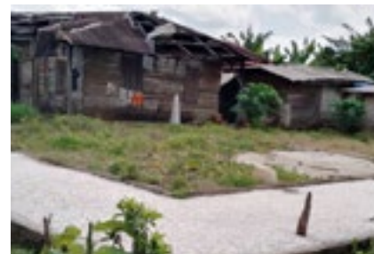
@Plan International damaged wooden shelters in the Southwest: Koupe Manigouba
