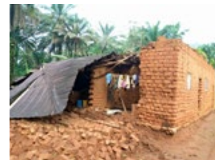
@INTERSOS Damaged Mudbrick Shelters in Bui Division Northwest
