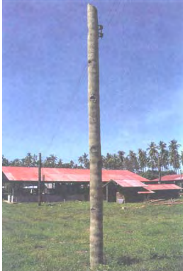
Photo 20: CCA-treated power pole
