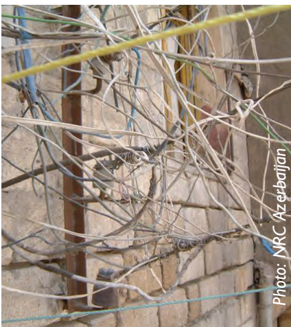
Wiring before upgrade
