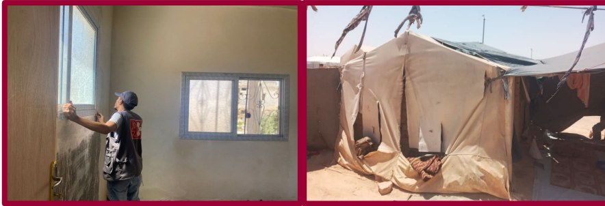
Left: Rehabilitation of damaged or unfinished housing in Dar'a - Neimeh, credit: PUI.
