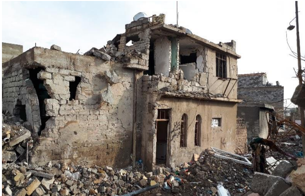
Category 3: severe damages, structurally compromised
