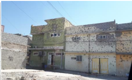
Category 1: minor damages to walls, doors and windows
