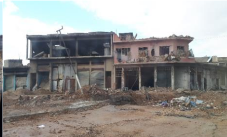
Category 2: major damages, structurally not compromised
