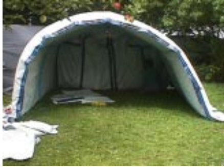
deformation of the shelter under the Self-weight of the mineral fibre roof
