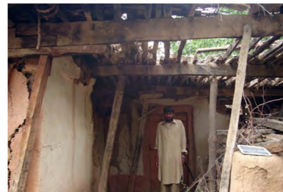
Traditional stone unreinforced masonry walling with heavy timber and mud roofs. The majority of this type of house collapsed completely.
