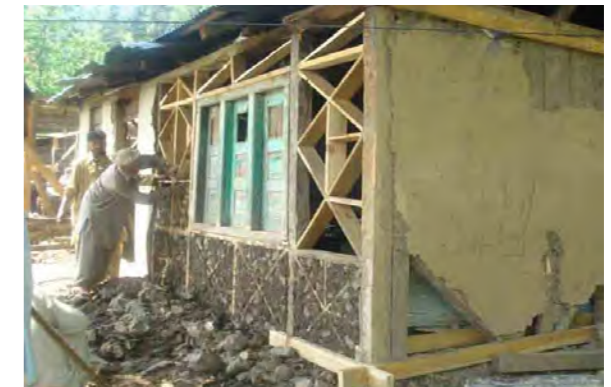
Demonstration sites included repair and retrofitting work as well as new construction sites.
