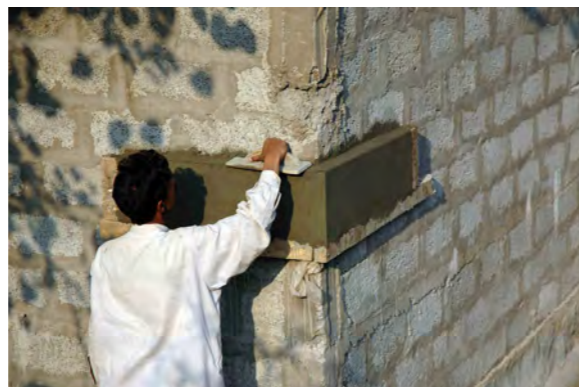
Mason plastering external corner stitch at a demonstration site. Simple solutions were promoted with standardised step by step advice for households.
