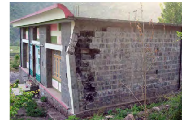
Reinforced concrete frame buildings were not designed or constructed adequately for earthquakes. Low levels of knowledge, skills or quality control.
