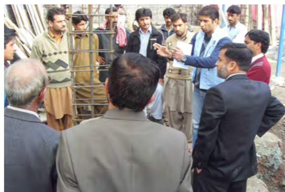
Training structural engineer explains construction defects to municipality engineers, contractors and local masons and steel fixers.
