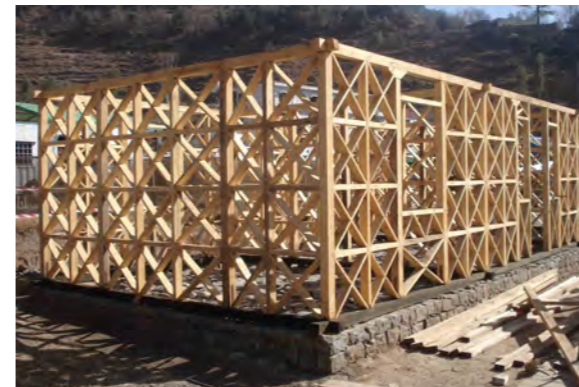
Dhajji house at HRC used for training and promotion at the resource centre.
