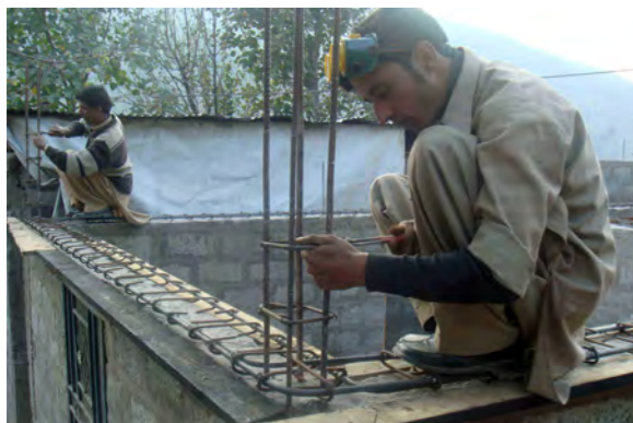
Technical support included master artisans like this UN-HABITAT steel fixer guiding on site at key stages in construction through practical assistance.
