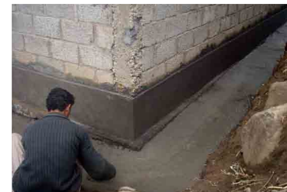
Plinth improvement and apron under construction, improving site drainage and durability of buildings to extend their lifespan, reduce dampness and increase hazard resistance.
