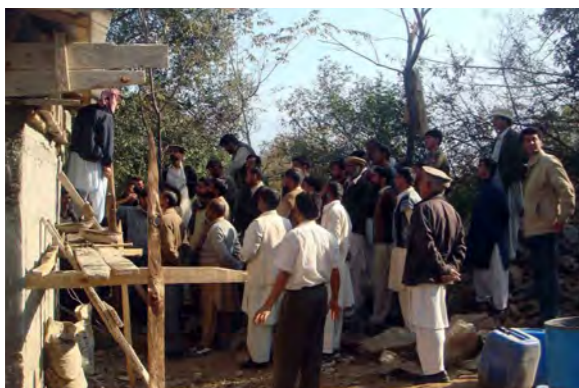
Community visit retrofitting demonstration site, increased skills and promotion were needed for retrofitting, site visits ensured better explanations.
