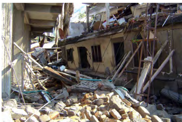
Damage in Muzaffarabad city centre, over 10,000 killed in city of around 130,000 persons, and extensive damage to public and private buildings.
