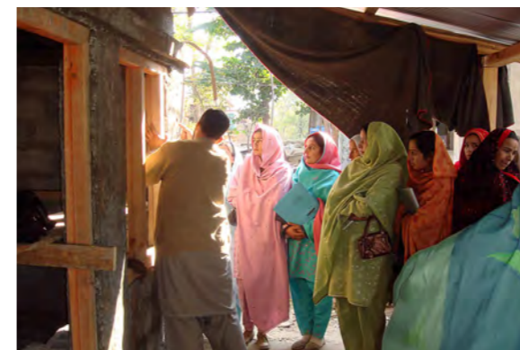
ERRA programme engineer explaining retrofitting measures to women's group. Women were important to plan the budgets and therefore investment in safety
