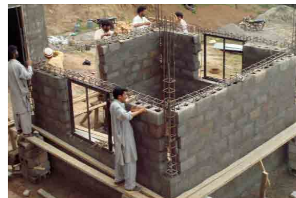
Training on a demonstration site. Many demo sites were left partially unfinished so the key reinforcement details were visible long term.
