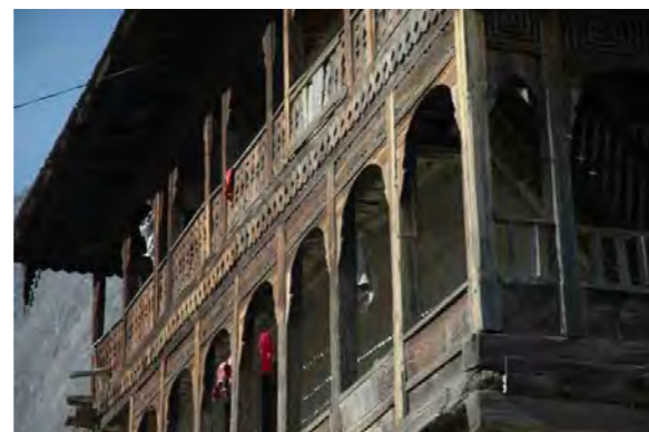
ERRA approved Leepa type construction for appropriate repair, revitalising conservation skills, safeguarding built heritage for future generations.
