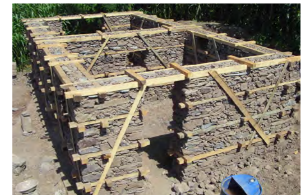
Bhattar construction in east Kashmir introducing an alternative technique in a remote area. Constructed by an experienced mason from another province.
