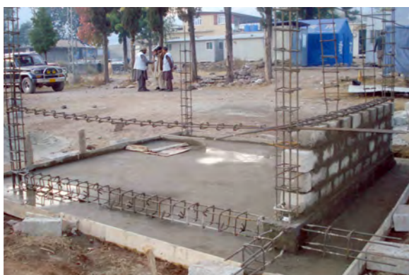
Demonstration construction at municipality offices and other locations in the city for training information and promotion of safer building.
