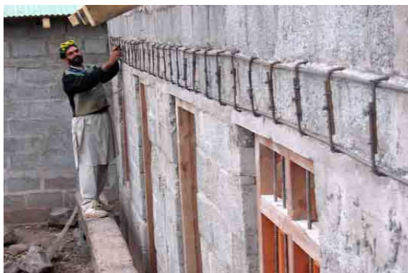
House with insufficient and discontinuous lintel is retrofitted with an lintel band, simple and affordable improvement with minimal disruption to the building.
