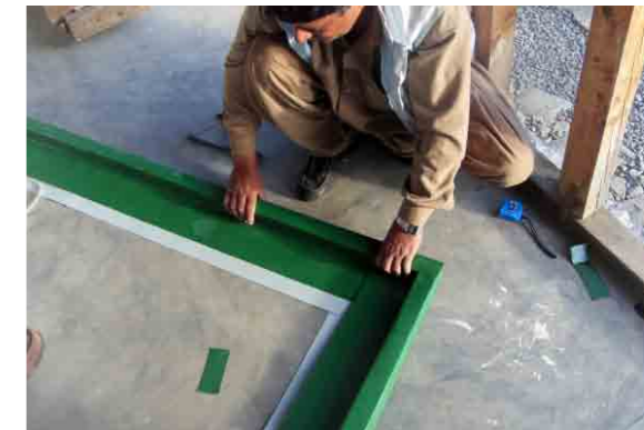
UN-HABITAT trainer demonstrating how to fabricate a corner section for the gutter for rainwater harvesting. Practical training to improve local practices.
