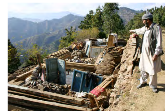
House owners present at site for damage assessment. No incentive for owners to increase damage to change from damaged to fully destroyed category.
