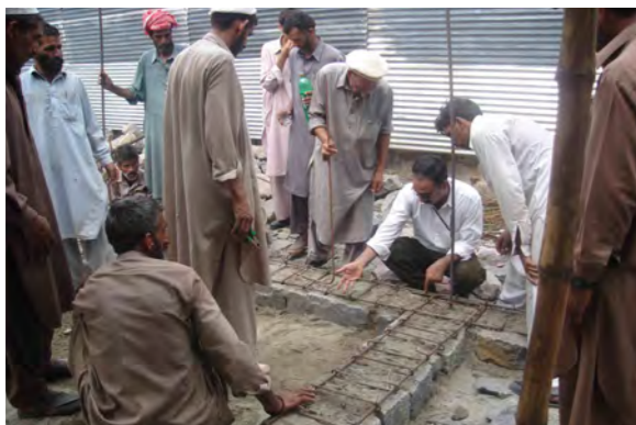
training for masons at Housing Reconstruction Centre. Training was also carried out at village level. The focus was on practical training to ensure understanding.
