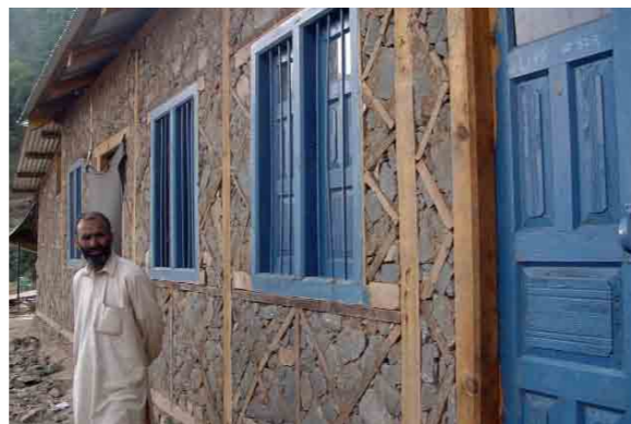
Improved local technology using locally available materials and salvage. Timber frame with stone and mud infill. ERRA approved technology feasible for many.
