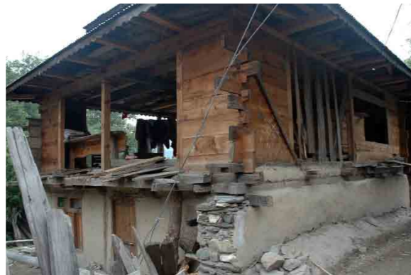
Repair and upgrading of traditional post and beam house, Leepa. These houses performed well in the earthquake, but minor damage needed appropriate repairs.
