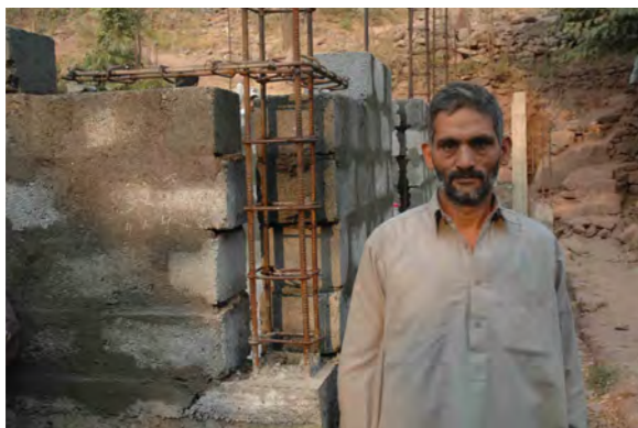
Mason in front of his own new home in confined masonry. Masons built their own houses very well from high earnings due to reconstruction business.
