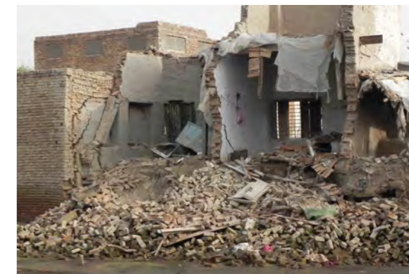
Monsoon flood 2010, ERRA teams carried out official technical surveys of housing types, damage and needs and prepared standards for reconstruction.
