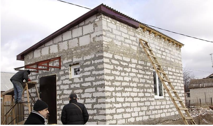
Luxembourg Red Cross project aimed at re-building completely destroyed houses in Sloviansk area © Jorge Valente / Luxembourg Red Cross | Semenivka, December 2015
