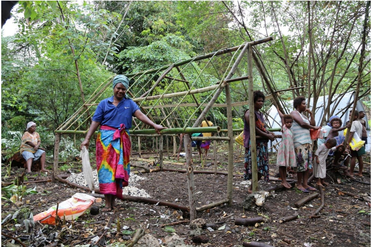
Bamboo frame under construction for a family displaced from a school at the start of the term, Nasawa
