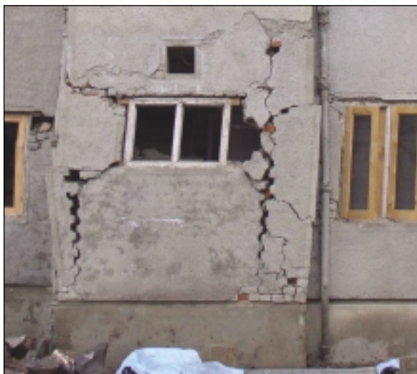
G4 damage cracks in brick wall
