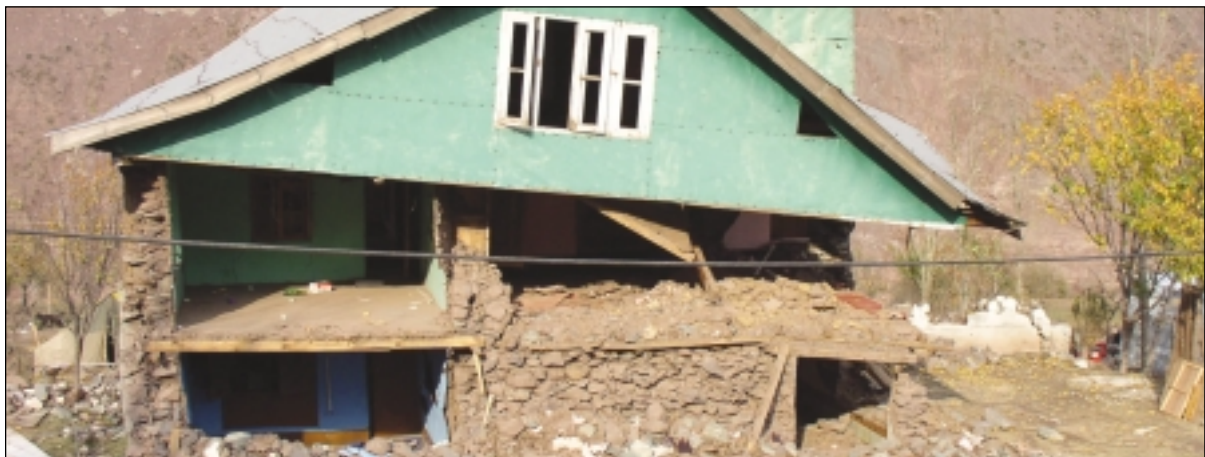
G5 damage in random rubble wall
