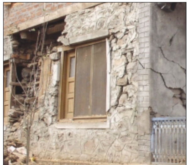
G4 damage in random rubble wall
