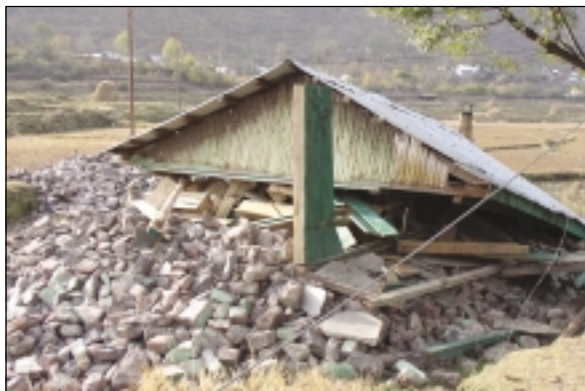
G5 damage, total collapse
