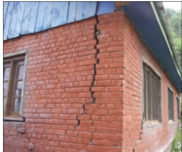
Damage due to poor wall-to-wall bonding
