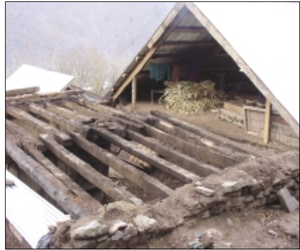
Damage to floor due to movement in support walls
