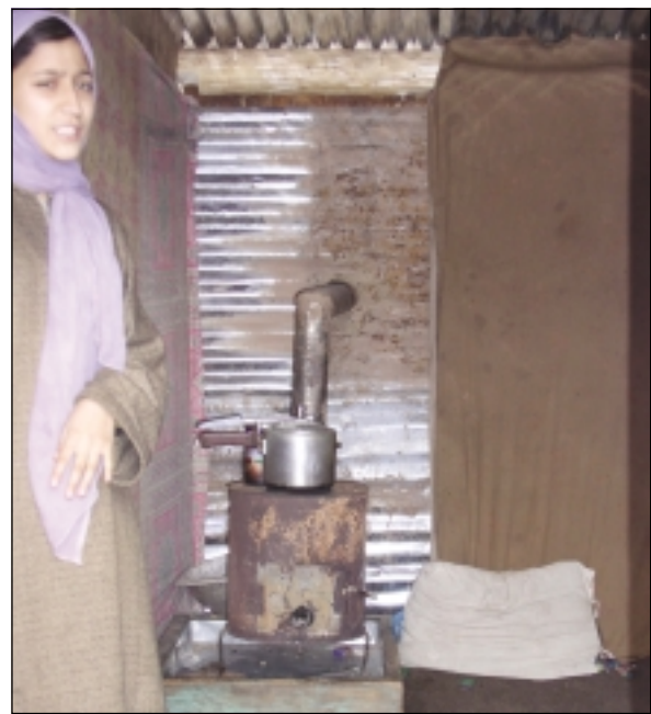
Bukhari space heater
