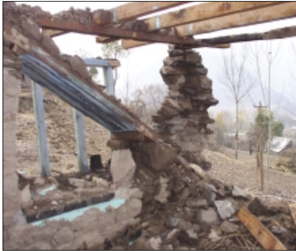
Snapping and collapse of timber floor joists
