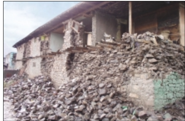
G5 damage in random rubble wall
