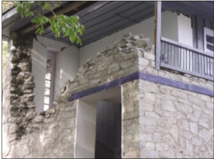
Partially collapsed wall
