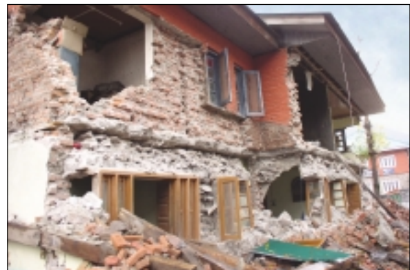
G5 damage walls heavily damaged, roof intact
