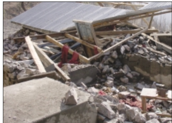
Roof destroyed due to wall collapse
