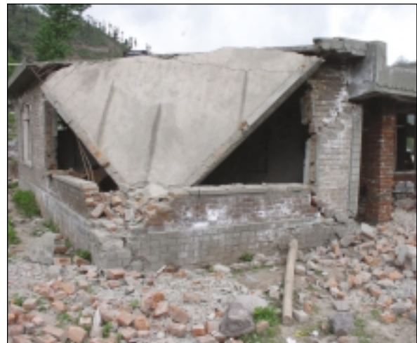
Collapse of a portion of slab due to collapse of some support walls
