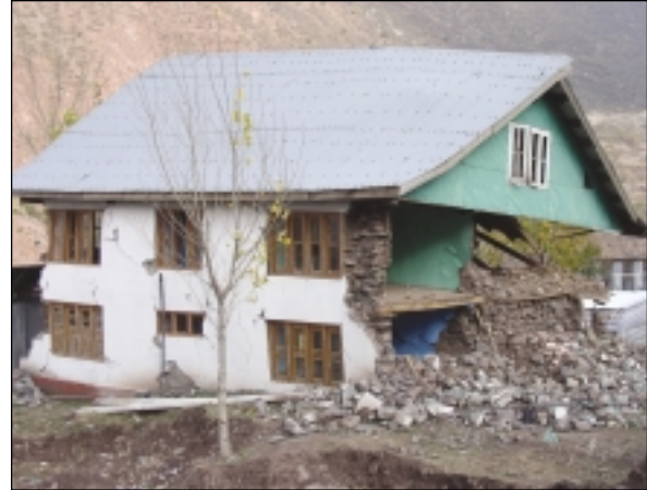
Roof needs to be jacked up and propped, followed by rebuilding of collapsed walls and repairing of damaged ones
