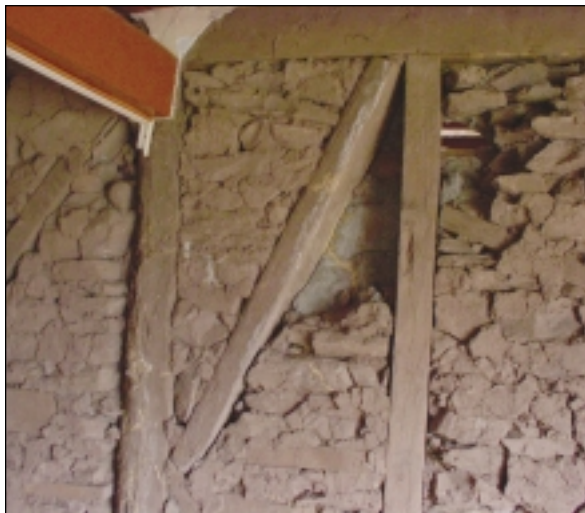
Small chunks of in-fill material falling out - the wall remains structurally safe
