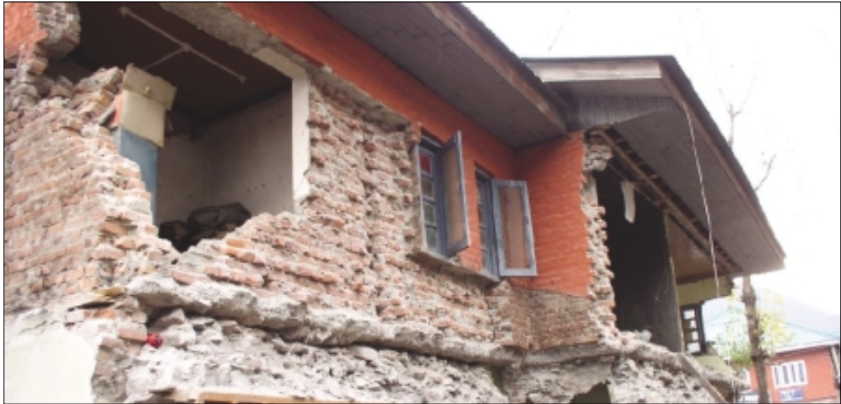
Wall damaged due to in-adequate bonding between brick masonry walls and roof deck
