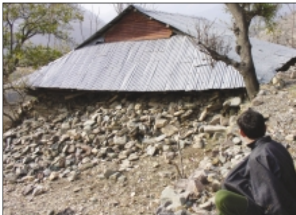
All walls collapsed but the roof is intact
