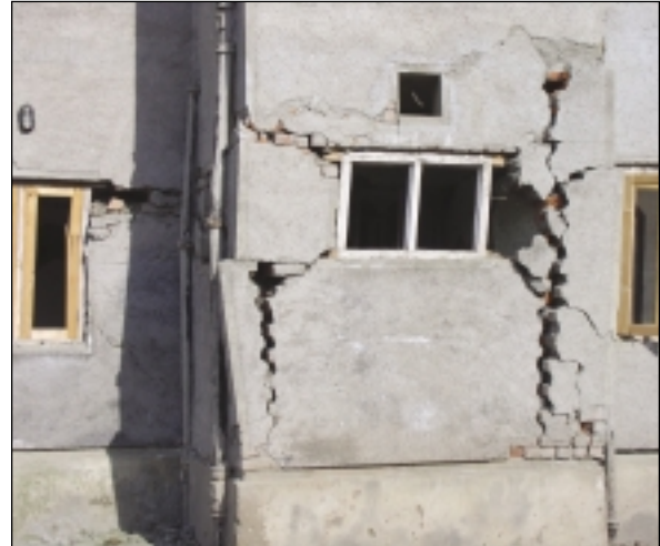
Damage due to inadequate in-plane tensile strength
