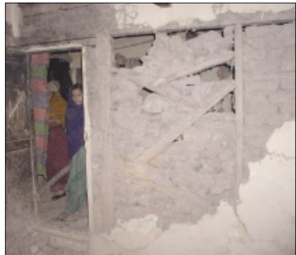
More chunks of in-fill material falling out - resulting in adverse affect to structural safety of the wall
