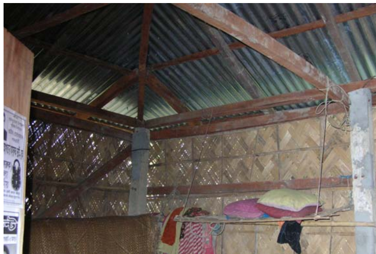
Note the use of precast RC columns, woven bamboo matting and corrugated metal roofing sheets
