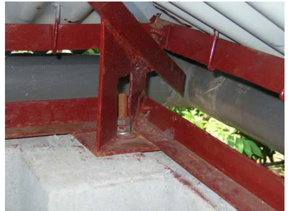
Good anchorage to reinforced brick pier. Note the use of J-hooks to secure the roof sheets.
