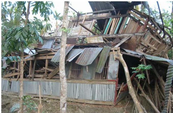
A well-built house destroyed by Cyclone Sidr
