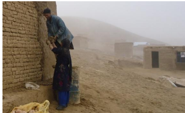
A widow helps with the plastering of her shelter. Soozma Qala, Saripul (Photo: ZOA)
