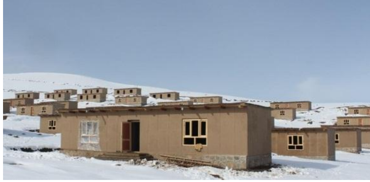
Construction delayed by winter in Abi Berek, Badakshan Province (Photo: Concern Worldwide)
