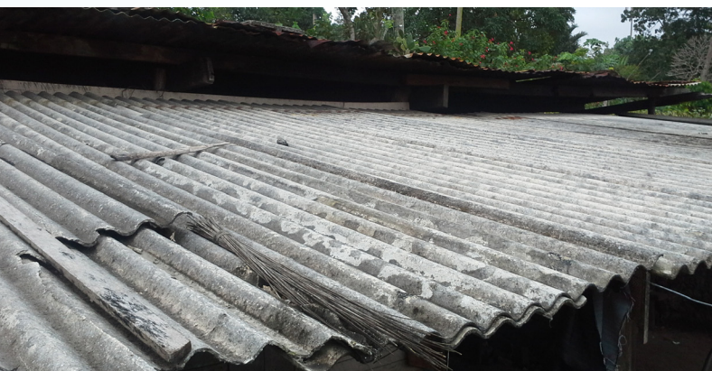
Corrugated asbestos cement roofing, pictured above on a building in Vanuatu, is relatively easy to recognise through visual inspection. Photo: PacWaste
