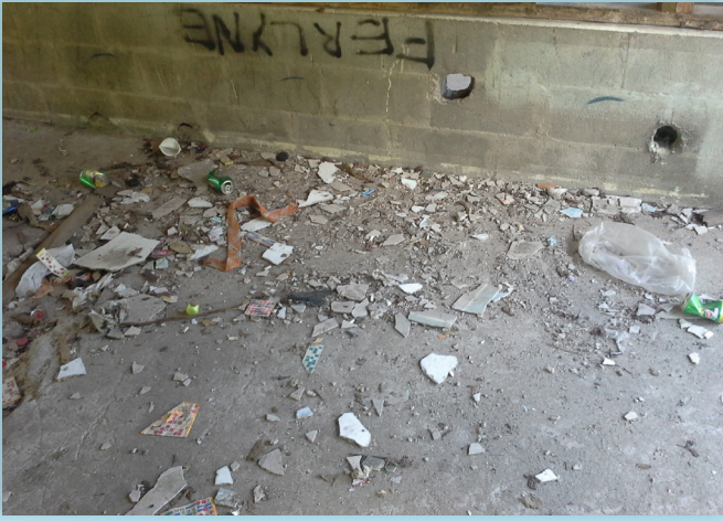
This vacant building in Nauru, littered with asbestos debris, appears to be frequented by young adults from the local community. Photo: PacWaste
