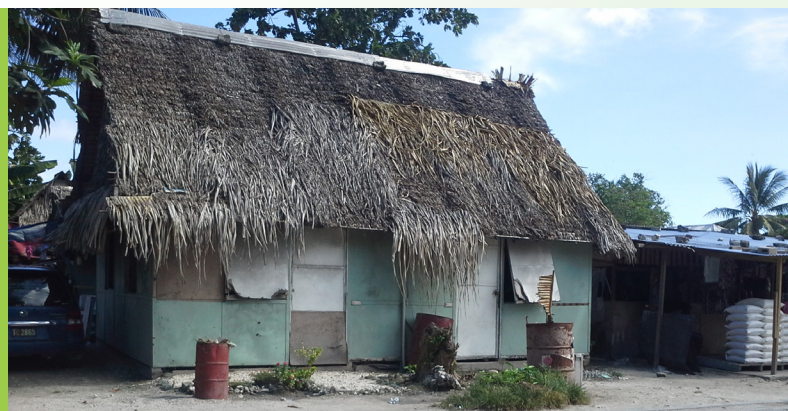
This typical residential dwelling on Tarawa, Kiribati may be built from asbestos cladding. However, testing would have to be undertaken to establish whether this is actually the case. Photo: PacWaste
