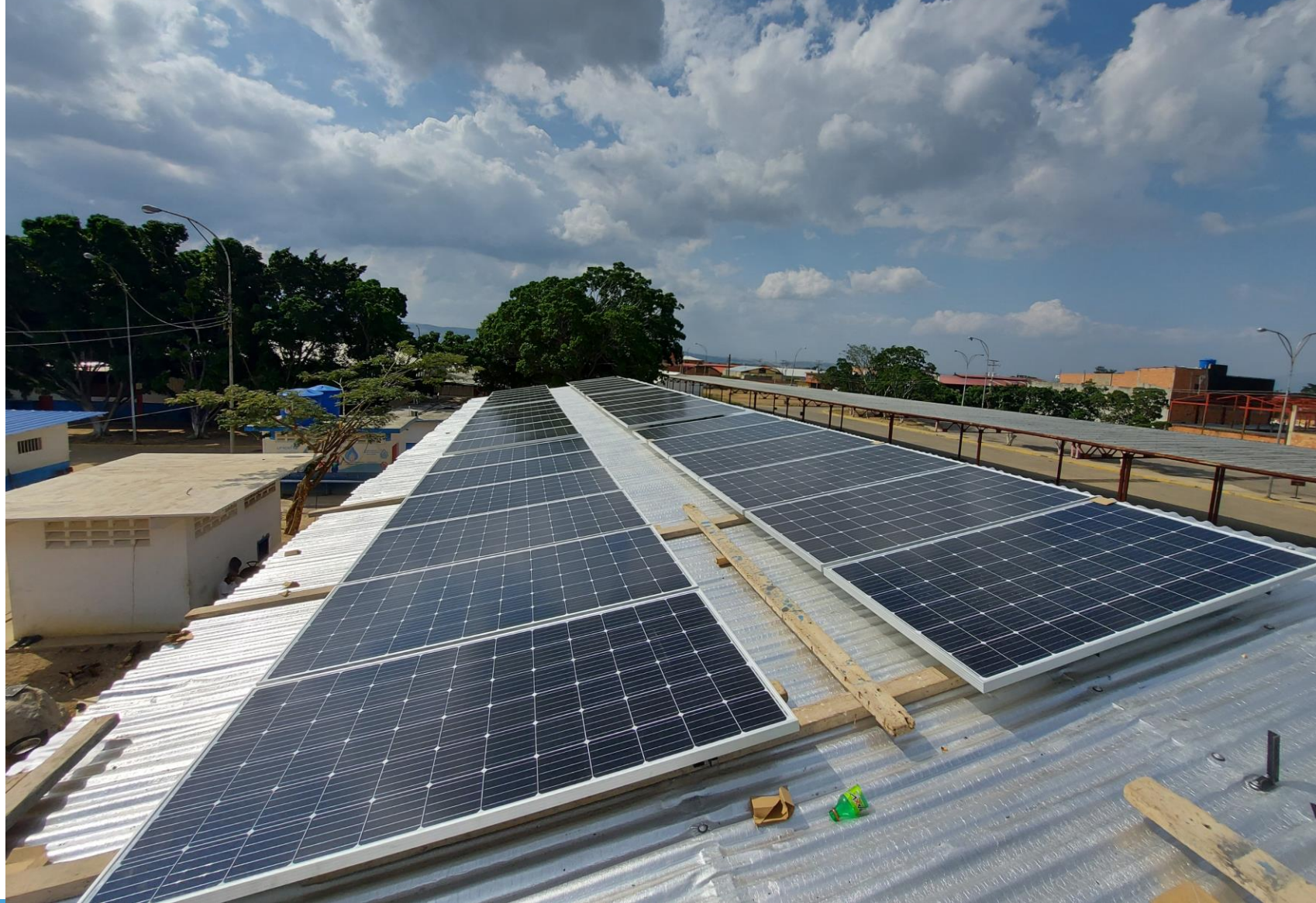
Photo: Photovoltaic installation at bus station, San Antonio, Táchira - UNHCR
