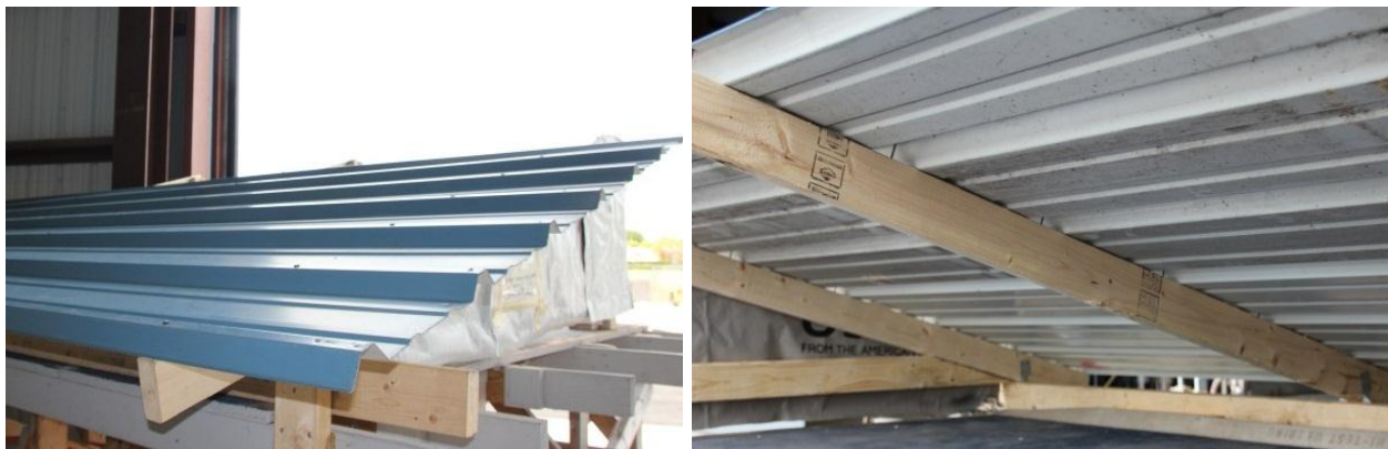
Figure 12 – 24-gauge PBR structural panel with no purlins or battens between rafters
