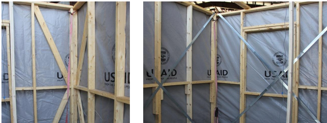
Figure 18 – Wall bracing techniques: corner diagonal wood braces (left) and metal strap diagonal X brace
