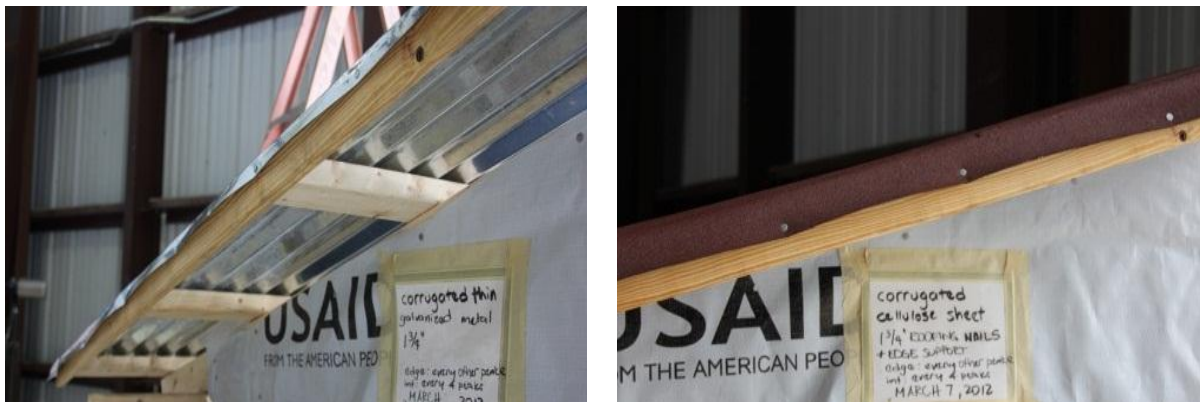
Figure 10 – Additional fascia board on purlin ends to provide additional fasteners on roof gable end
