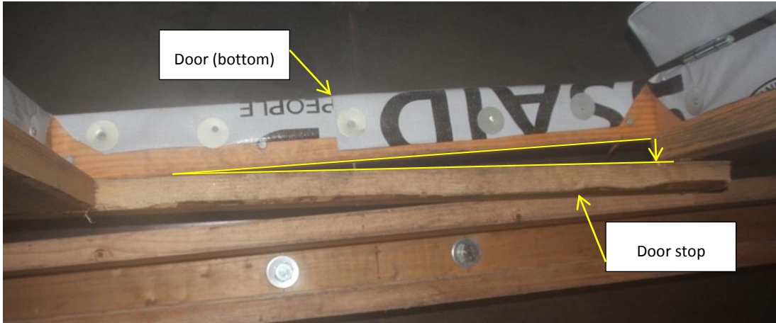
Figure 6 - Bottom door stop pulled-out
