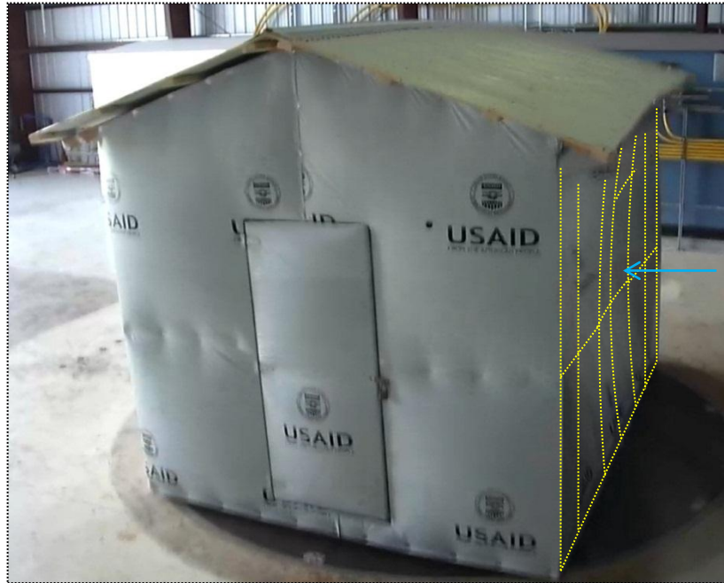
Figure 9 - Windward wall deformation at 0° angle of attack and 110 mph
