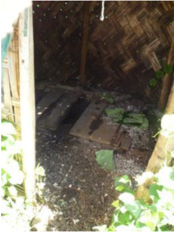
Figure 17: Latrine floor utilizing timber. The design of the latrine floor is flexible; it need only be able to support the plastic floor plate
